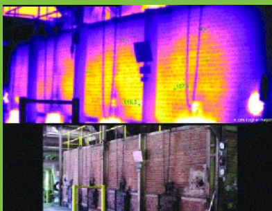
Check for abnormal hot spots indicating refractory insulation breakdown.
